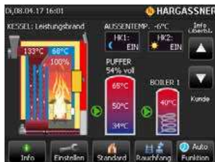
Boiler in Full-Load: Display shows a working boiler. HWT and Accumulator are being loaded already. Heating Circuits ensure required temperature in each living-area.
